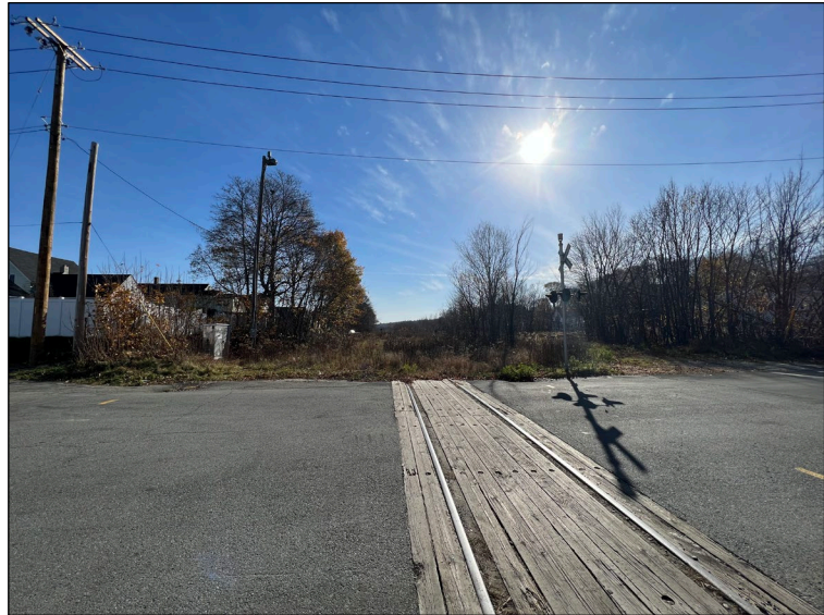
This photo shows the Elm Street railroad crossing in Millinocket. The track leads to One North industrial park. The track, crossing and protection devices will be rehabilitated under the Project.
